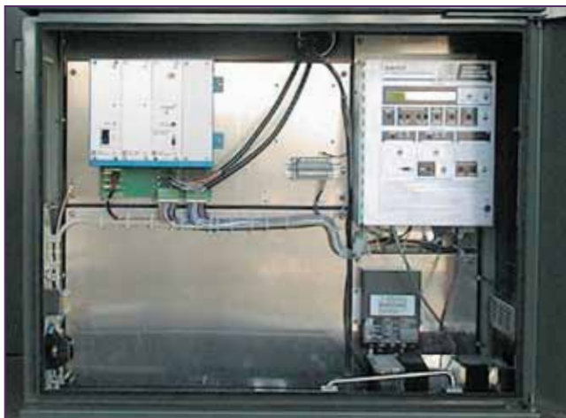
Remote Supervisory Vista UDS with 5800 Series Switch Control.
