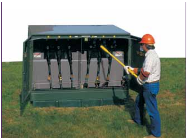
Figure 3. Operation of typical dead-front gear can be awkward and time-consuming.
