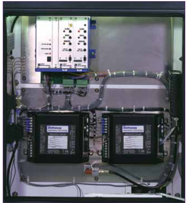
Details of low-voltage compartment of Remote Supervisory Vista UDS Model 422.
