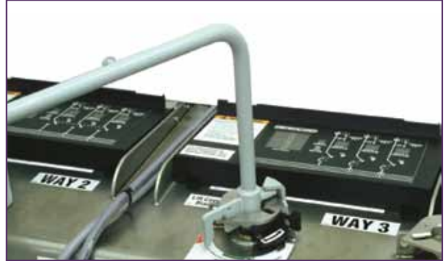
Figure 1. Opening load-interrupter switch (or fault interrupter).
